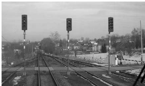
Fig. 3 Station interlocking plant
